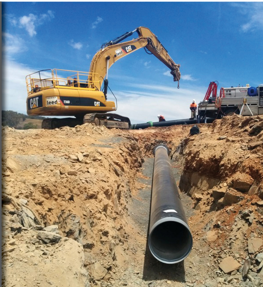
The 39 km Macquarie River to Orange Water Supply Project connects Orange’s Suma Park Dam to the Macquarie River, ensuring water security for Orange.
